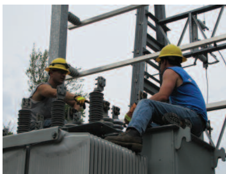
GETTING READY FOR THE MOVE: Linemen Chad Phillips, left, and Todd Molyneux prepare the Laporte transformer for its move.
