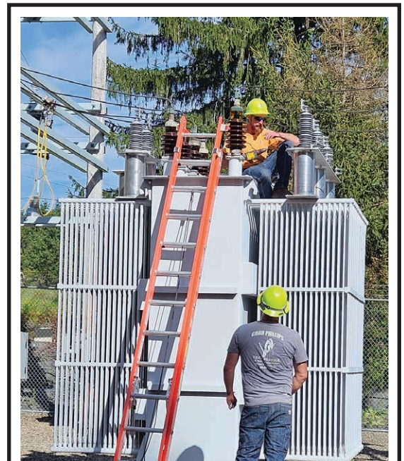
OUTAGE PREVENTION: Linemen Chad Phillips, standing, and Alex Laudermilch installed new lightning protection on our substation transformer in Dushore during the fall. This system improvement helps protect our equipment from failure in the event of a lightning strike. Thanks for the good work, guys!
