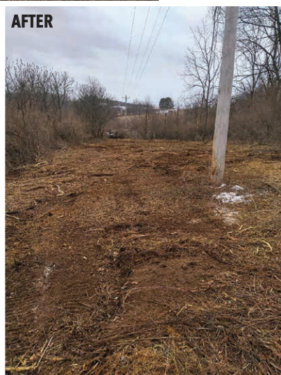
BEFORE AND AFTER: Contracted crews from Spako's Tree Services have been busy clearing miles of rights of way. This makes access to our lines easier for crews and lessens the chance of a tree or limb coming down on lines.
