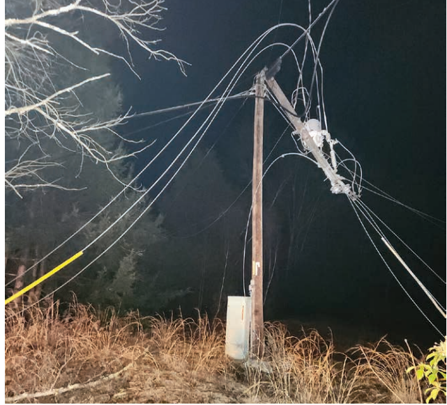
WIND DAMAGE: A windstorm swept through our service area this past spring, snapping utility poles and trees.
