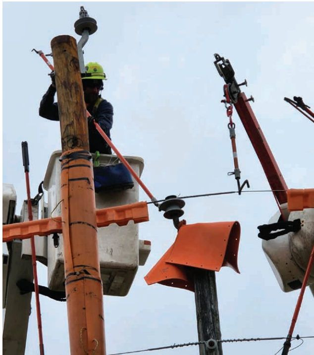
ALL IN A DAY’S WORK: SCREC crews work on establishing lines to a new pole.
