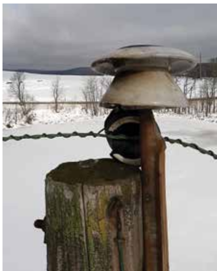
HIDDEN PROBLEMS: Not all causes for an outage can be readily seen. A broken insulator resulting in an outage can take a great deal of time to locate, especially at night.
