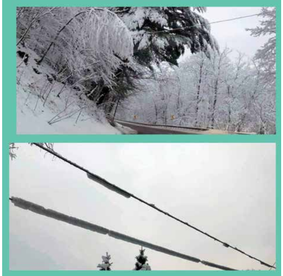
TEMPERATURE MATTERS: It's amazing how the difference of a few degrees can affect outages. With temperatures hovering around 32 degrees, a heavy wet snow fell causing area-wide outages Jan. 3. Outages can also occur after a storm if power lines "bounce" when the snow falls off, causing them to hit other lines.
