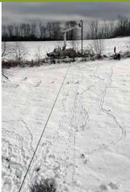
HARD AT WORK: Co-op line crews are made up of dedicated employees who work long hours, often in poor weather conditions, to restore power to members when outages occur.
